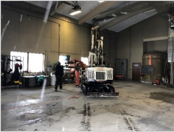
Exhibit 3-7: Discovery Drilling stages drill rig in ARFF garage prior to advancing boring B-IW-19 through CR-ARFF-1.
